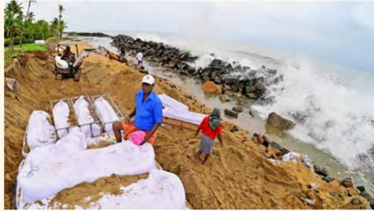
Concrete bags being filled with sand for placement against coastal erosion in Ernakulam district. (File photo for representation) | Photo Credit: H VIBHUJ
